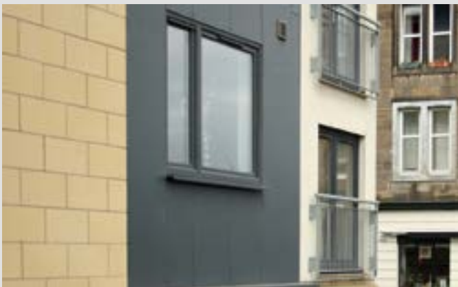
Too many materials The cladding, blockwork and render and their detailing used at this development would not now meet the Council's expectations for appropriate quality.
