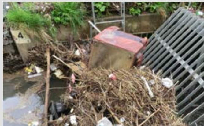
locked up culvert
